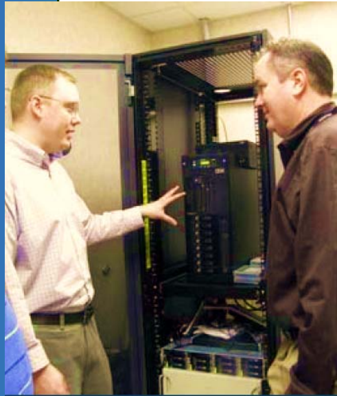
Kannapolis City Schools’ technology technician John Allen inspects a server with Todd Shanley, IT Manager for Cabarrus County.
